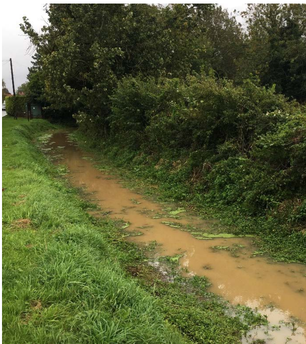
Figure 1: Example of the watercourse after maintenance has been completed. This view is looking downstream from Thorpe Road Bridge.
